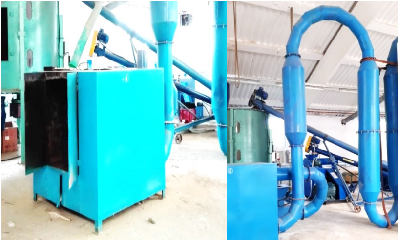
Figure 6 Drying installation (Industrial Park Cenei)
