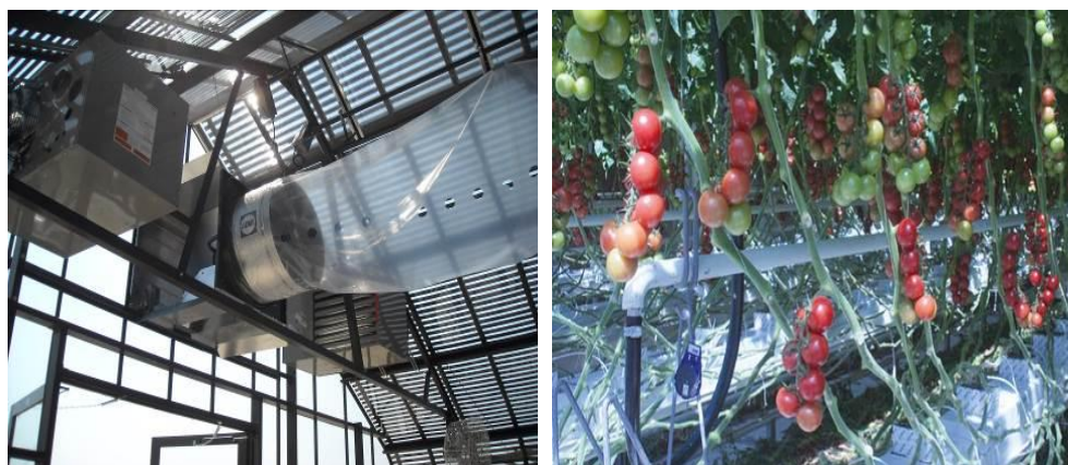
Figure 3 Jet fan heating (left) and hot water heating with pipes (right)
