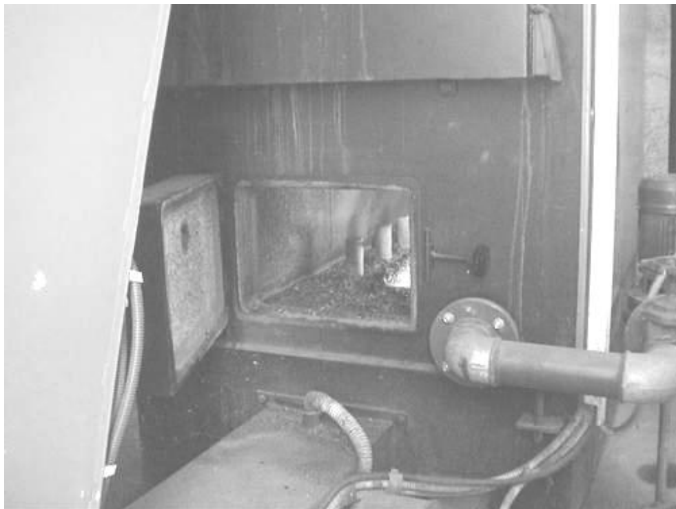
Figure 3. The boiler's furnace
